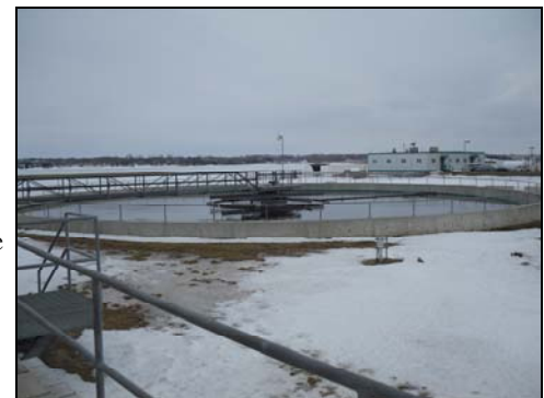
TANKS CONTAINING CLEAN WATER (SECONDARY CLARIFIERS)
